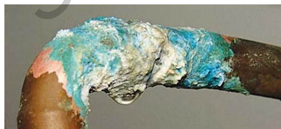
fig-18: Corrosion of copper
